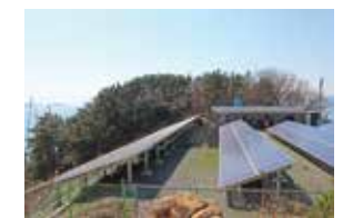
Front view of Modular Hybrid energy power supply system of Jam-do, KC Cottrell
